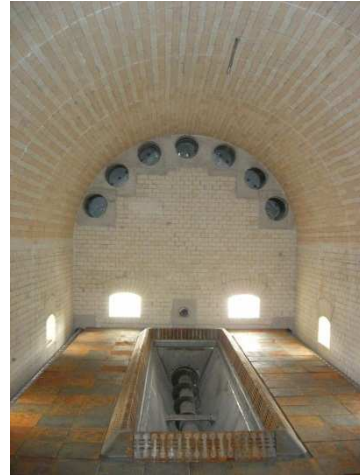
Semi wet biomass screw furnace
