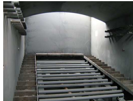
Wet biomass screw furnace
