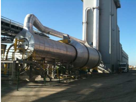
Natural gas combustion furnace
