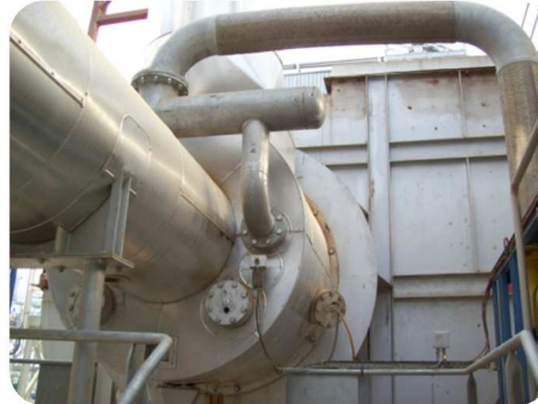
Natural Gas Burner
