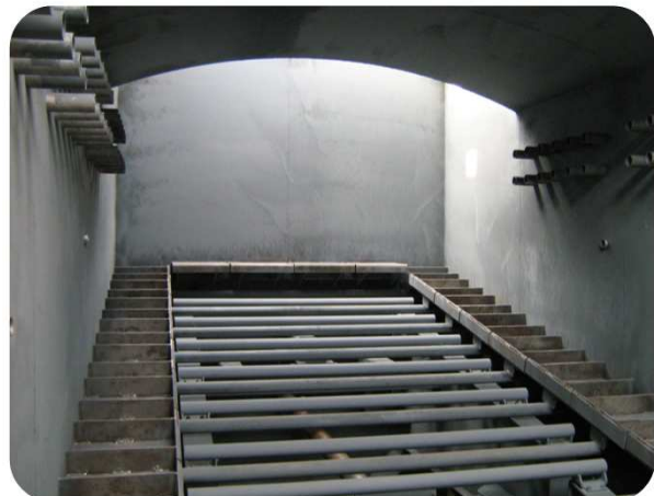
Wet Biomass Grate Furnace
