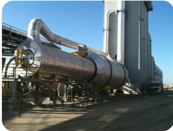
Natural Gas Combustion Furnace
