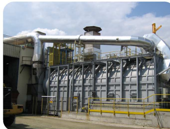
Semi- Wet Biomass Furnace
